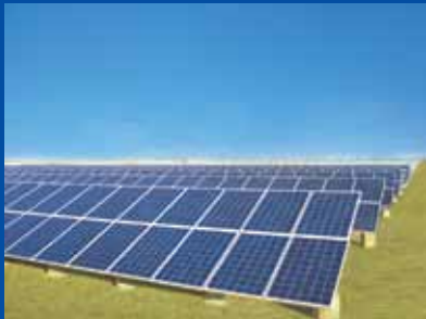
25 MW Solar Plant, Sural EPC by Sterling & Wilson
